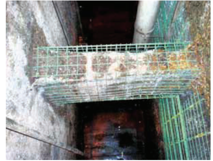
After surface preparation, rebar was installed for all areas requiring more than 1 in. of concrete repair.
