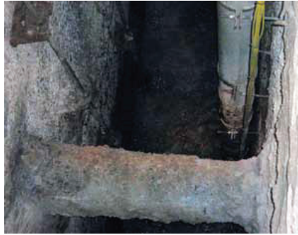
This initial Jersey City wet well inspection photo shows the significant concrete deterioration on the walls and support beams, down to the large aggregate.
