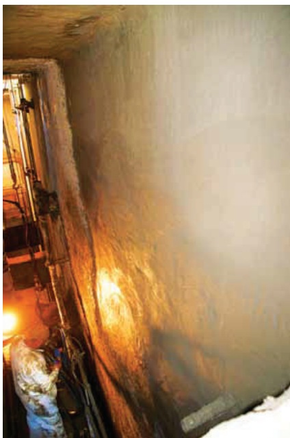
Substrate resurfacer is applied via wet shotcrete, allowing high-build installations over the rebar areas.
